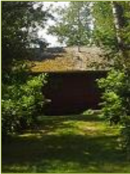
Figure 21. Debris build up on roof
