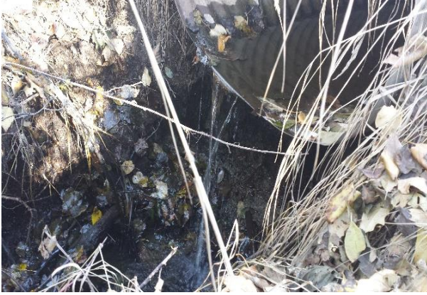
Photo 11: Crossing 2 culvert outlets showing gap that blocks fish passage.
